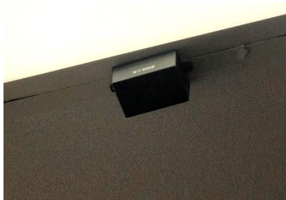
SONR Echo Box: Installed In-Store (on ceiling)
